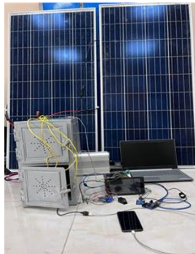
Figure 18: Overall Integrated System installation
